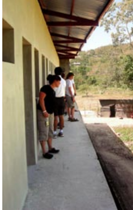
Members of the work group from St. Thomas Church, Fort Washington, Penn. are standing where a balcony will be added, contemplating what they can do to help finish the new Our Little Roses mountain retreat facility called Our Lady of the Roses Retreat House and Weeks-Schilling Training Center.
